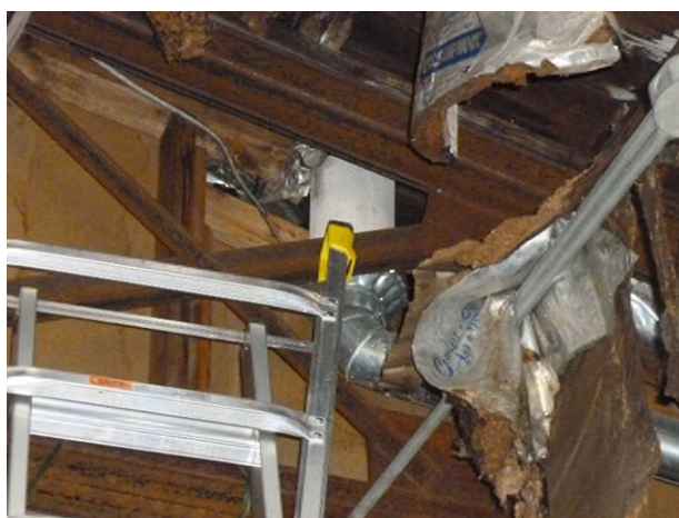
HA-7: Gray Vent Stack Insulator
