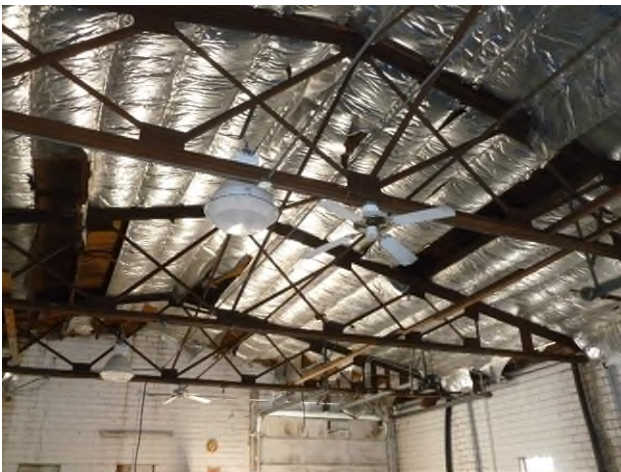
HA-20: Ceiling Deck Insulation
