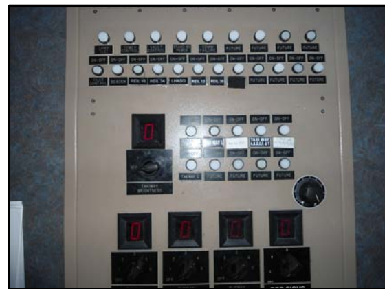
EXISTING L-821 PANEL
