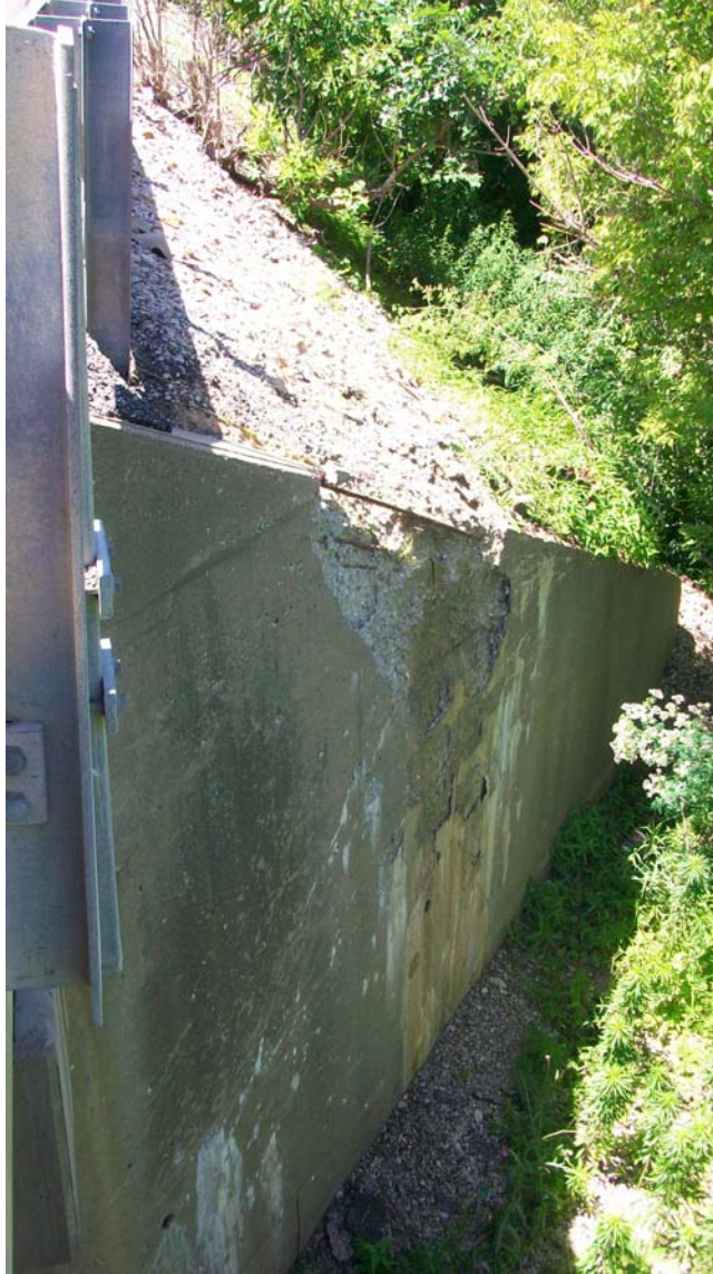
Photo 6 North West Wing Wall with Reinforcement Exposed
