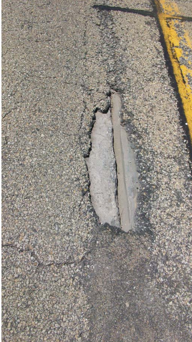
Photo 14 Exposed Substructure near Center of Bridge
