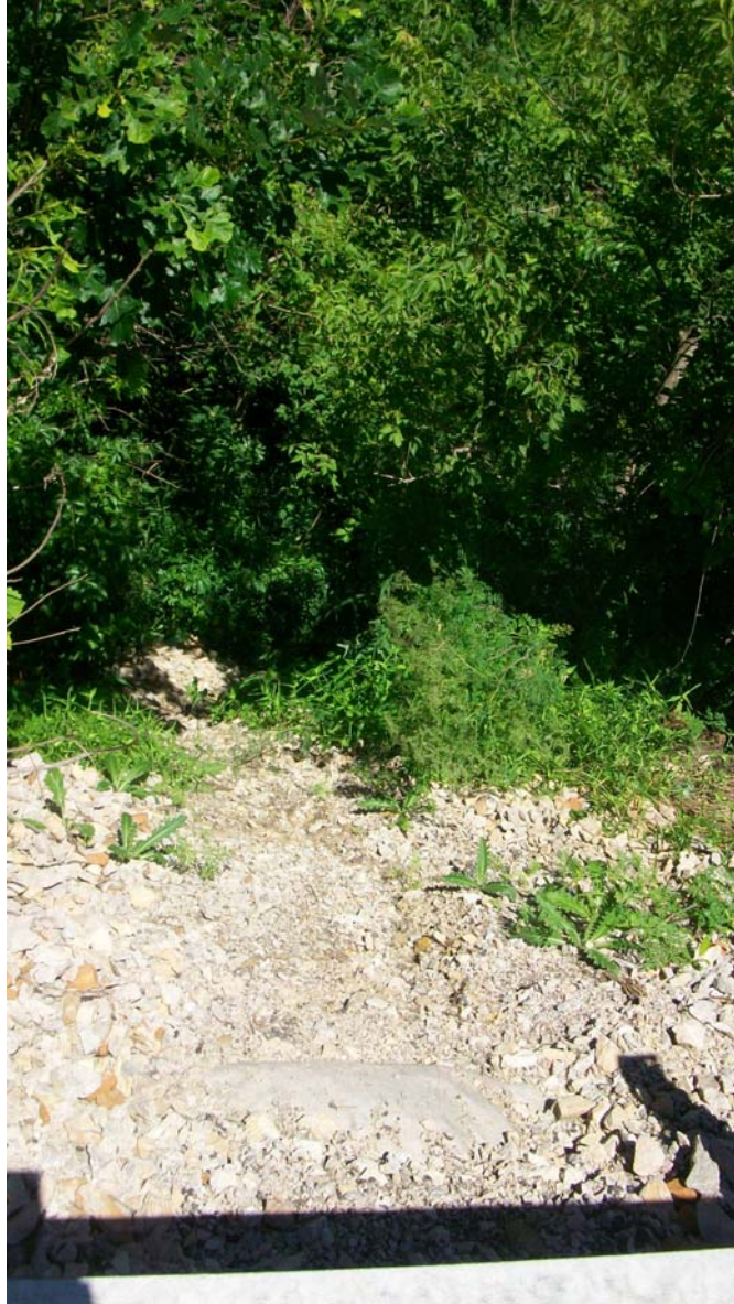
Photo 5 Erosion on North West Ditch Showing Erosion and Exposed Fabric
