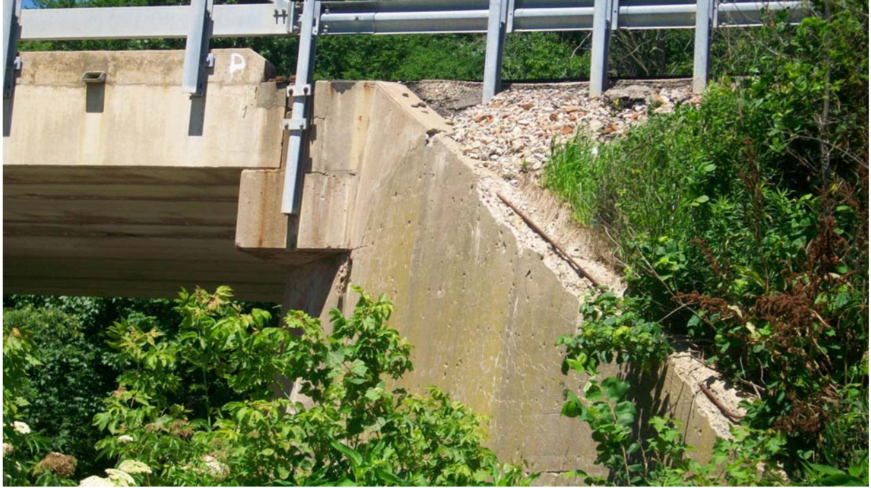
Photo 3 South East Wing Wall
