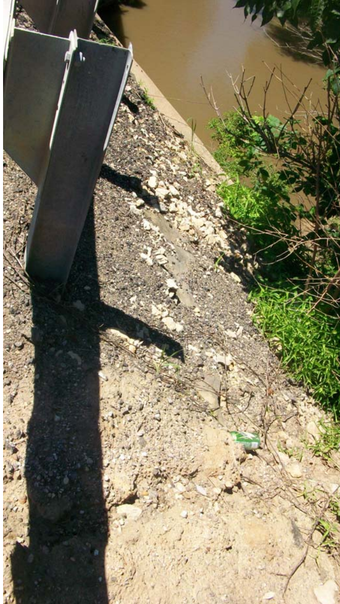
Photo 9 Erosion above North East Wing Wall Showing Exposed Fabric
