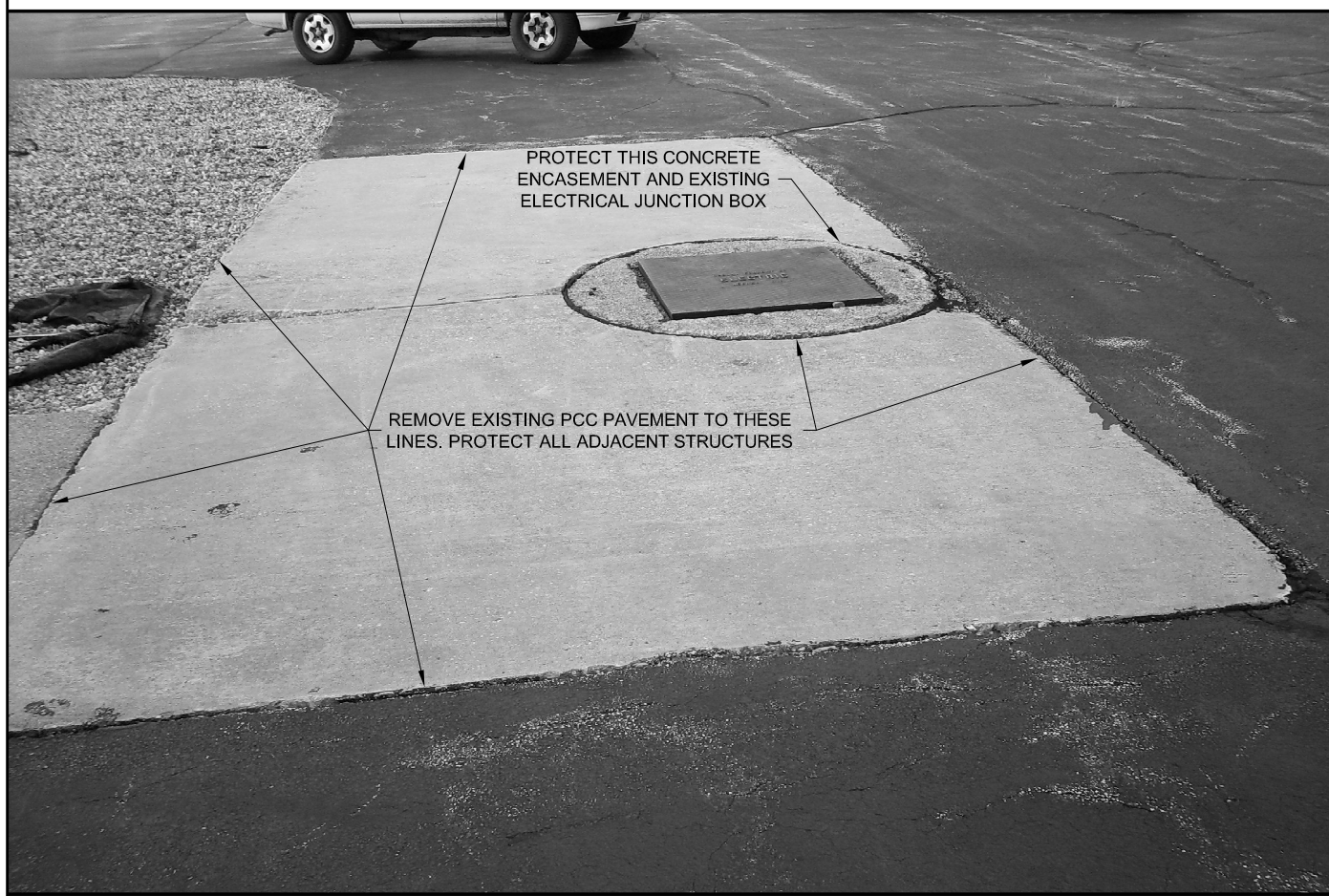
GOLF RAMP - EXISTING ELECTRICAL JUNCTION BOX
