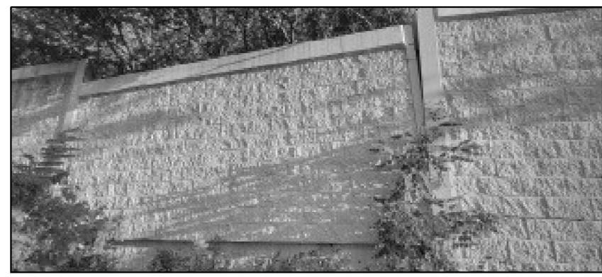
LOCATION 17 I-290 WB EAST OF IL-56 (BUTTERFIELD RD.) REPLACE 20' X 14' NOISE WALL
