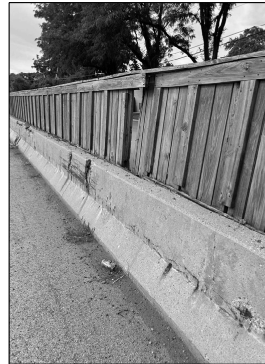
LOCATION 22 IL-83 SB ABOUT 0.75 MILES NORTH OF IL-64 REPLACE 4' X 6' WOOD NOISE WALL
