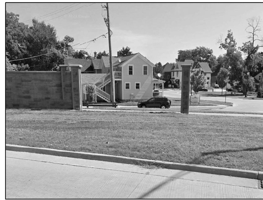
LOCATION 29 IL-31 ABOUT 0.40 MILES SOUTH OF IL-62 (ALGONQUIN RD.) REPLACE APPX. 7' BY 12' PRECAST CONCRETE NOISE WALL
