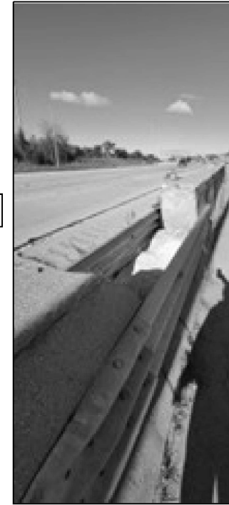
LOCATION 10 I-290 WB AT INDIANA ST. REPLACE 13 FT OF MEDIAN BARRIER WALL
