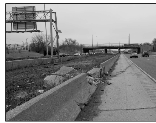
LOCATION 6 I-94 NB MEDIAN ABOUT 0.10 MILES WEST OF MATIN LUTHER KING DR. REPLACE 23 FT OF SHOULDER BARRIER WALL
