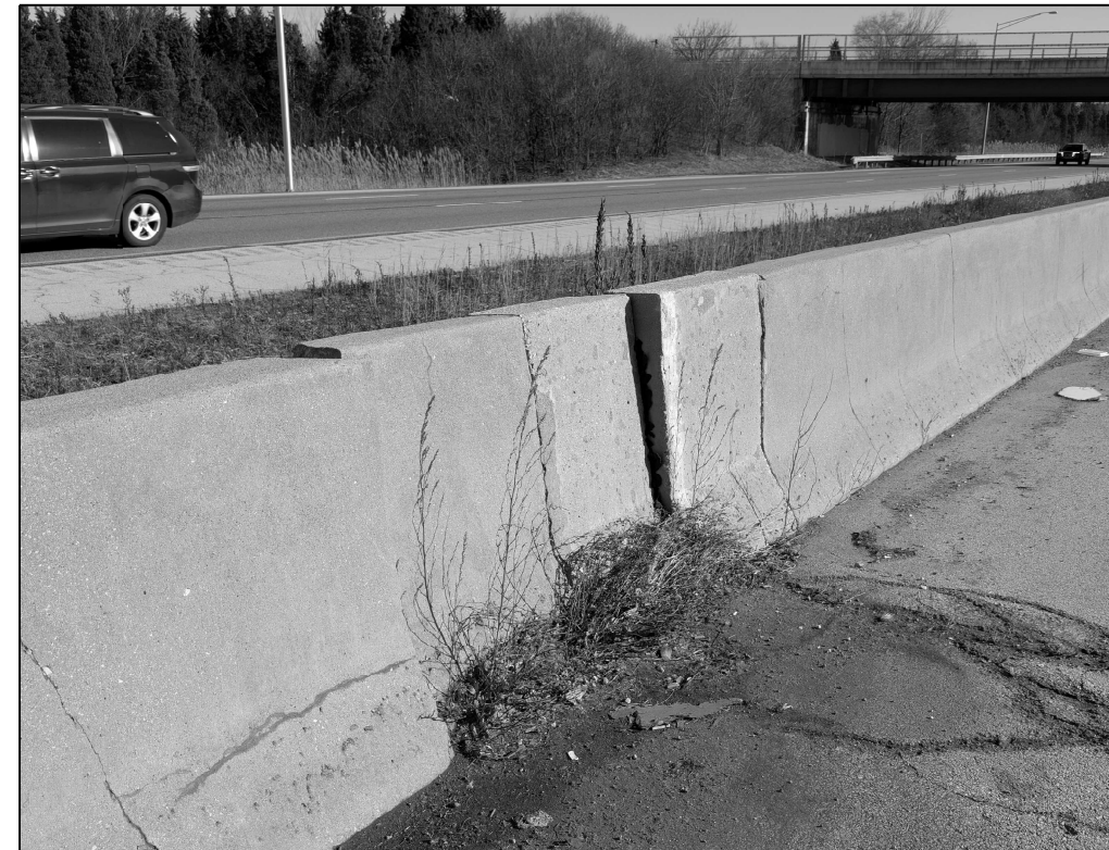
LOCATION 12 I-290 EB ABOUT 340' WEST OF MILL RD. REPLACE 4 FT OF SHOULDER BARRIER WALL
