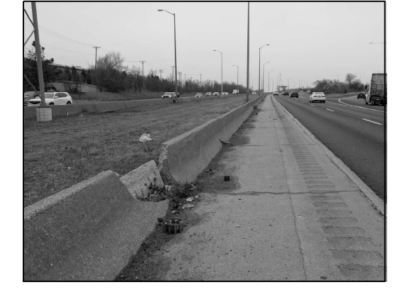
LOCATION 9 I-94 SB ABOUT 130' EAST OF COTTAGE GROVE REPLACE 8 FT OF SHOULDER BARRIER WALL
