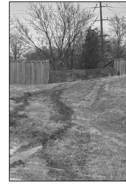
LOCATION 27 IL-83 NB NEAR BURLINGTON AVE./RAILROAD REPLACE FIVE SECTIONS 8' X 12' EACH WOOD NOISE WALL WITH POSTS
