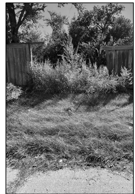
LOCATION 24 IL-83 NB ABOUT 0.17 MILES SOUTH OF US-34 (OGDEN AVE.) REPLACE TWO SECTIONS 9' X 6' EACH WOOD NOISE WALL WITH POSTS
