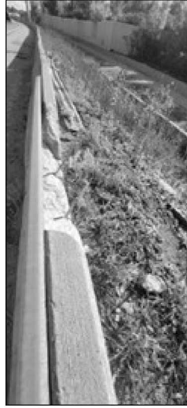
LOCATION 4 I-290 E.B. 0.25 MILES WEST OF WOLF ROAD FULL DEPTH BARRIER WALL REPAIR REPLACE 8 FT OF SHOULDER BARRIER WALL
