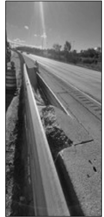
LOCATION 11 I-290 WB NEAR US-20 WB FLYOVER REPLACE 18 FT OF MEDIAN BARRIER WALL
