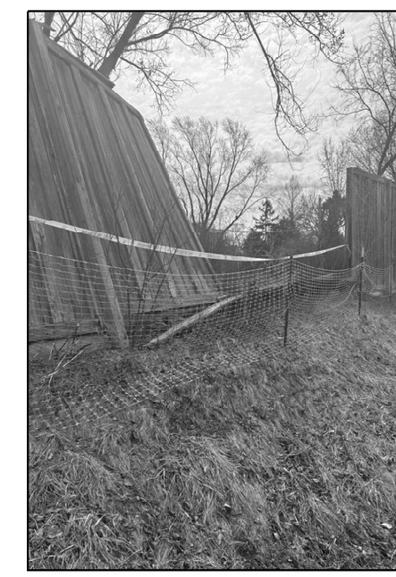
LOCATION 26 IL-83 NB ABOUT 0.35 MILES NORTH OF US-34 (OGDEN AVE.) REPLACE EIGHT SECTIONS 8' X 12' EACH WOOD NOISE WALL WITH POSTS
