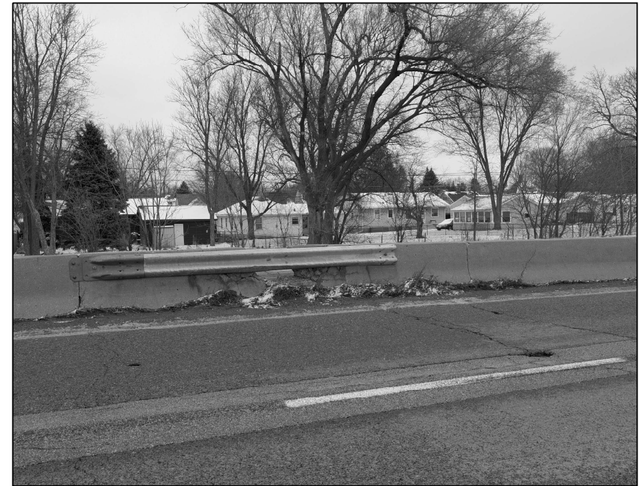
LOCATION 13 US-20 APPX. 0.3 MILES WEST OF IL-31 REPLACE 14 FT OF MEDIAN BARRIER WALL
