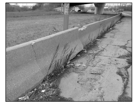
LOCATION 7 I-94 NB JUST SOUTH OF 100TH ST. REPLACE 23 FT OF SHOULDER BARRIER WALL
