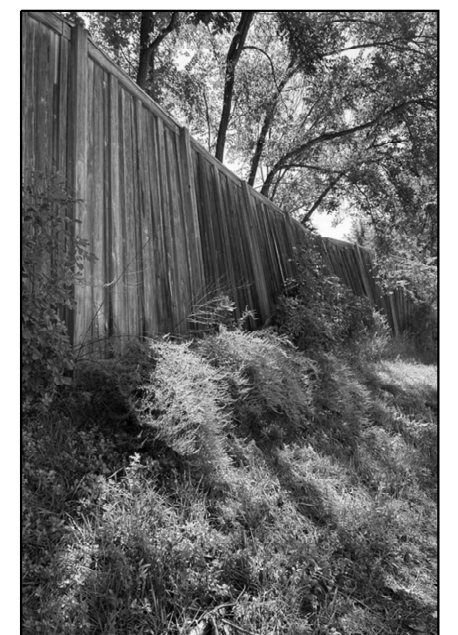
LOCATION 25 IL-83 NB ABOUT 0.30 MILES SOUTH OF US-34 (OGDEN AVE.) REPLACE EIGHT SECTIONS 9' X 12' EACH WOOD NOISE WALL WITH POSTS
