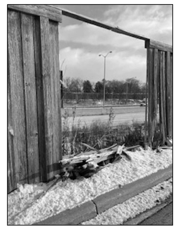
LOCATION 30 I-290 EB ABOUT 0.15 MILES EAST OF EMROY AVE. REPLACE ONE SECTION 12' X 10' WOOD NOISE WALL
