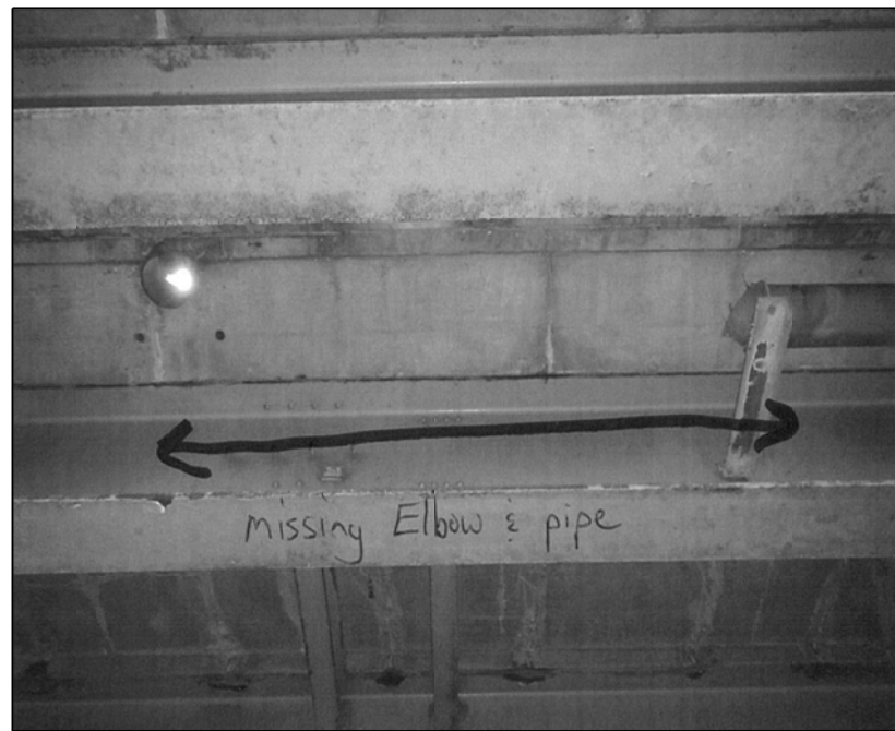
016-0128 PHOTO #1 MISSING DRAINAGE PIPE SECTION
