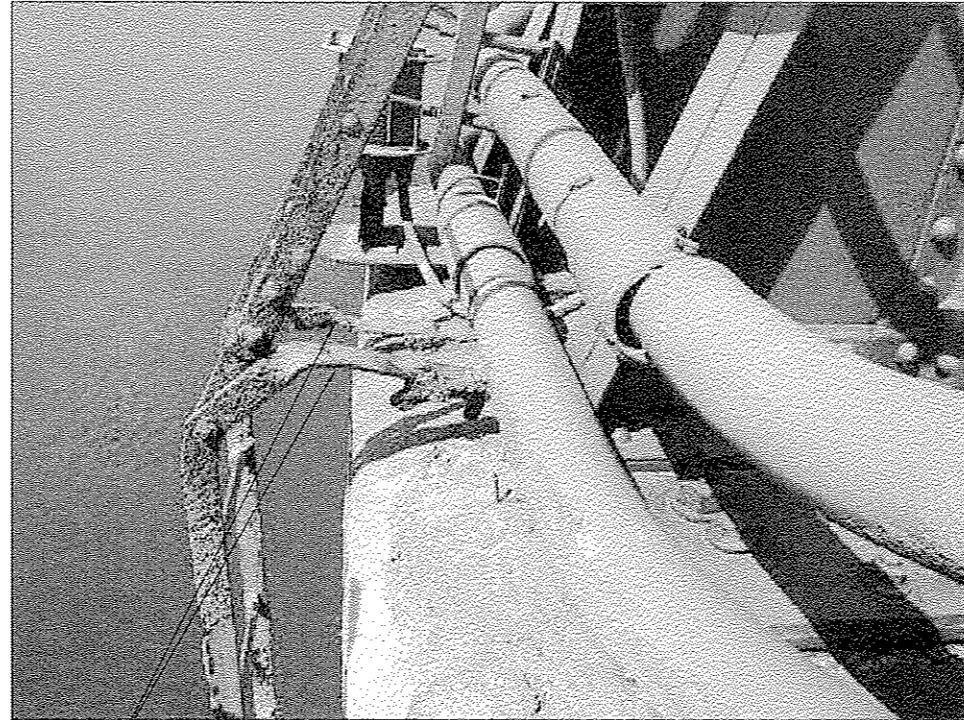
ITEM 612 Ladder at S. end of Pier 9
