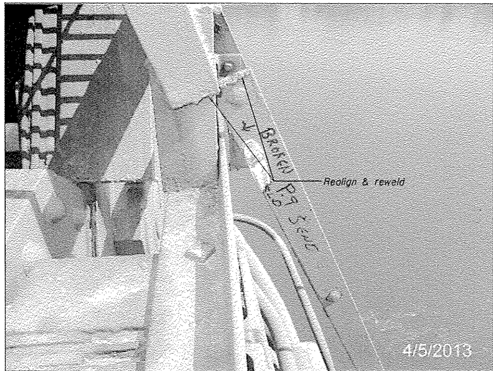
ITEM 612 Ladder at S. end of Pier 9
