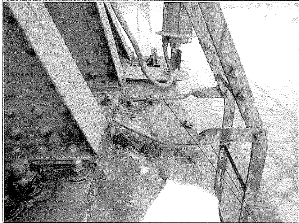
ITEM 611 Ladder at N. end of Pier 9
