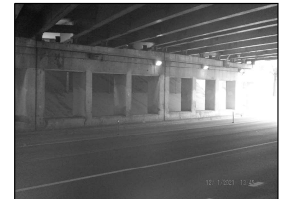
EXISTING LIGHTING: PIER 1 (Looking Southeast)
