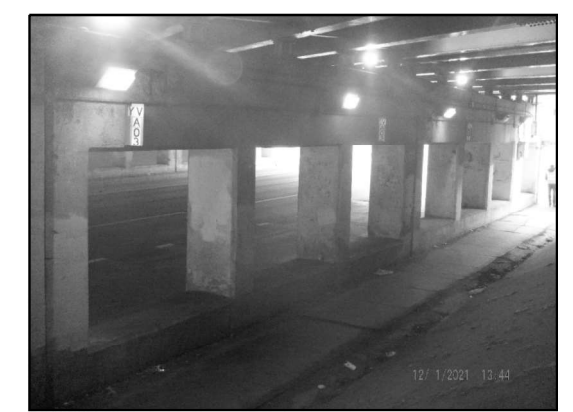
EXISTING LIGHTING: PIER 2 (Looking Southeast)
