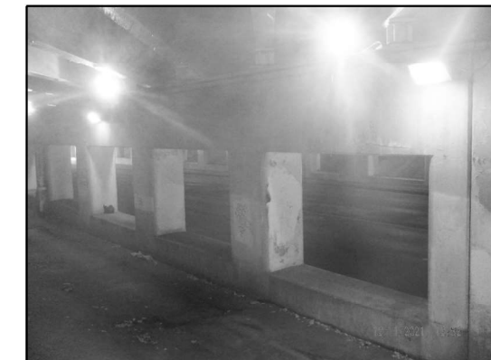
EXISTING LIGHTING: PIER 1 (Looking Southeast)
