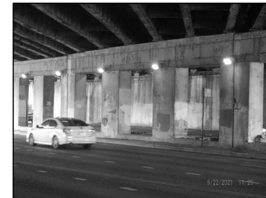
EXISTING LIGHTING: PIER 2 (Looking Southeast)
