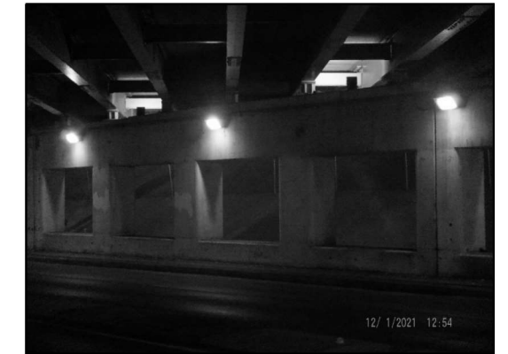
EXISTING LIGHTING: PIER 2 (Looking Southeast)
