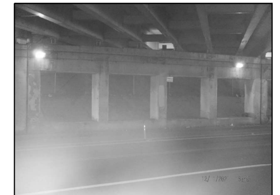
EXISTING LIGHTING: PIER 1 (Looking Southeast)
