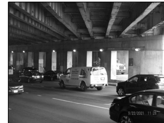
EXISTING LIGHTING: PIER 2 (Looking Southeast)
