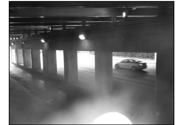
EXISTING LIGHTING: PIER 1 (Looking Southwest)
