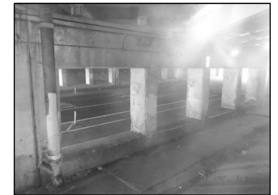
EXISTING LIGHTING: PIER 2 (Looking Southeast)
