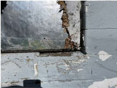
HA-9: White Exterior Window Caulk
