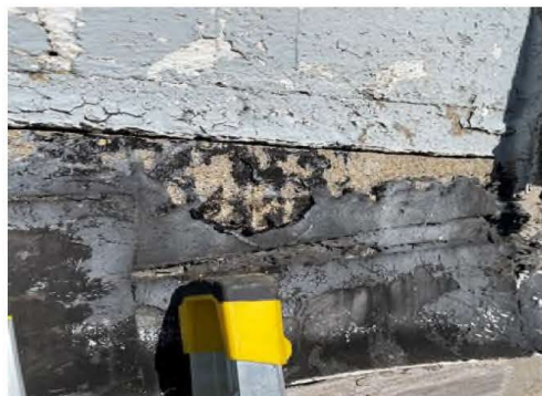
HA-12: Black Tar on Flashing
