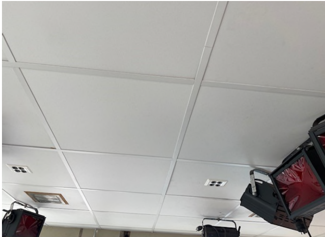
HA-8: White Gypsum Board Ceiling Panels
