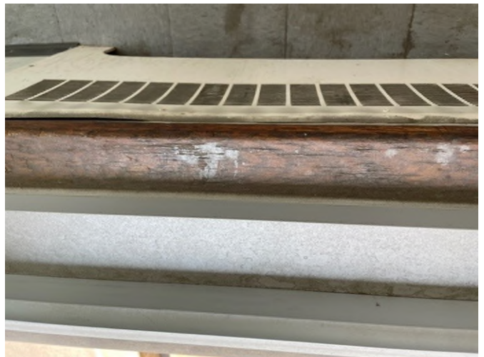
HA-7: White Window Frame Caulk
