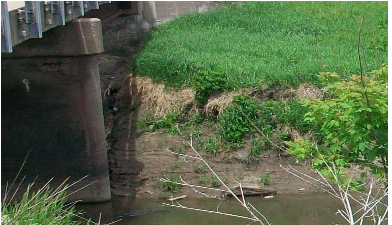
Picture # 4 Northeast creek bank
