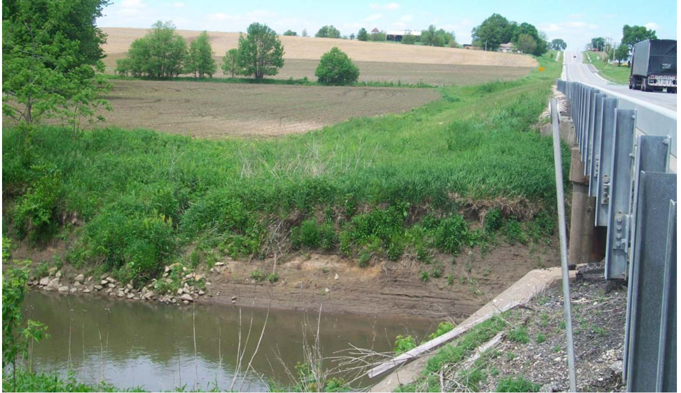
Picture # 1 Northwest ditch
