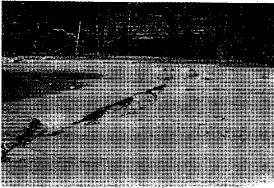
High Severity Shattering Type Blowup
