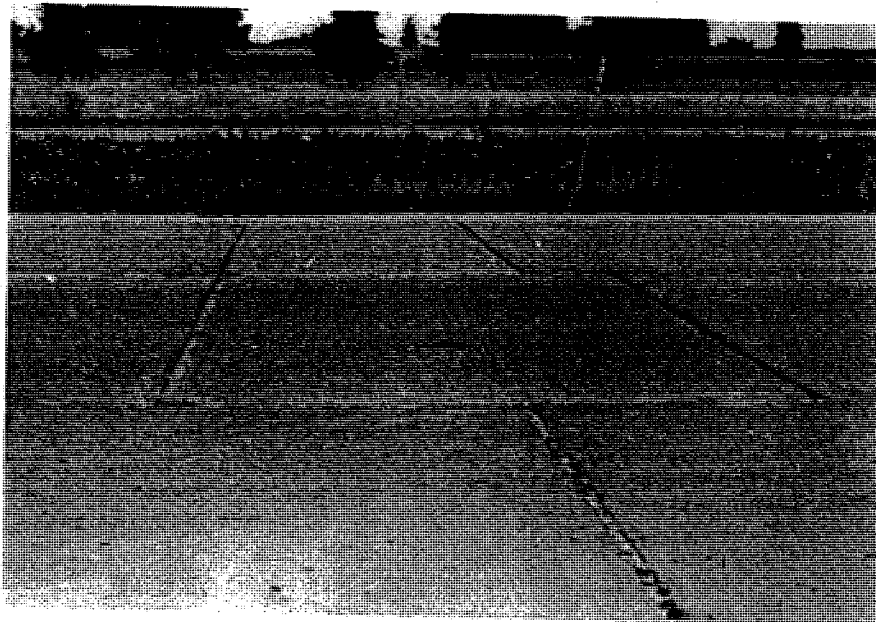
Low Severity PCC Concrete Patch Deterioration
