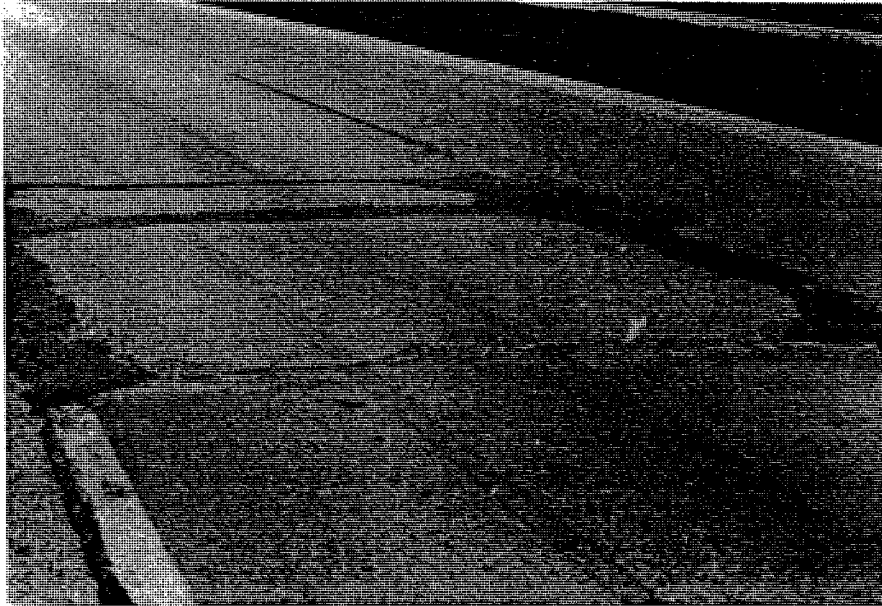
Medium Severity PCC Concrete Patch Deterioration
