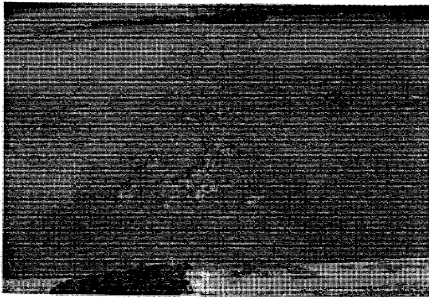
Medium Severity D-Crack
