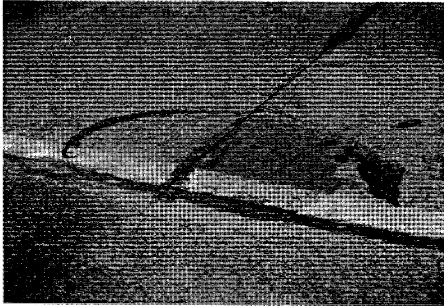
Low Severity Corner Break
