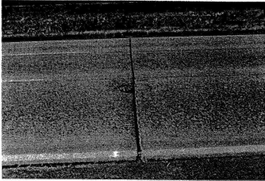
Low Severity Spalling
