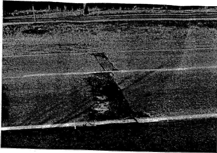
High Severity Joint Load Transfer System Associated Distress
